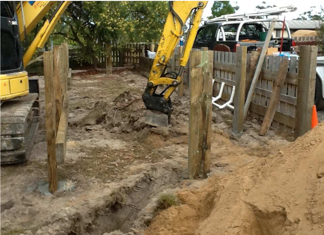
Plate 2 (below). Ripping soil over the base of the basic module. Filter sand in right foreground.
