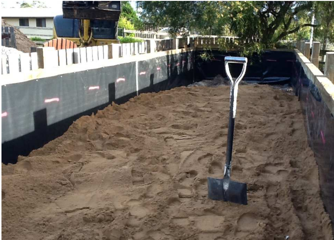
Plate 5 (above). Placement of filter sand. Lay in nom. 100mm layers; walk over to slightly compact, especially against plastic around edges.
