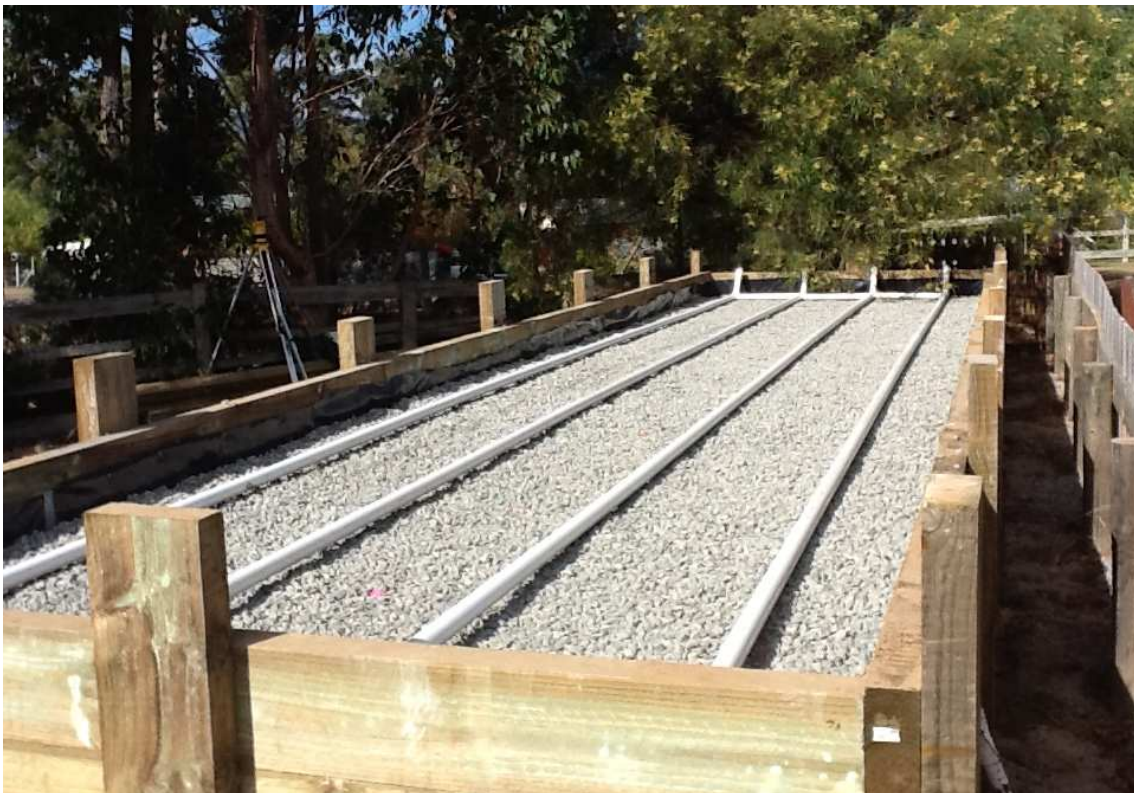
Plate 8 (below). Grid of 40mm Class 9 UPVC pipework in place, with raised inspection openings at far end.
