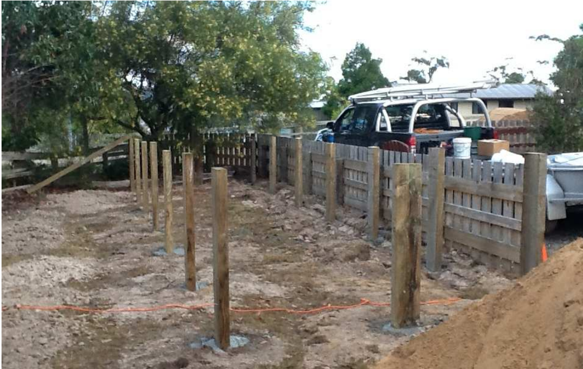
Plate 1 (above). Posts (200 x 75mm sleepers) at no more than 1.5m centres concreted in holes at least one third of their height.
